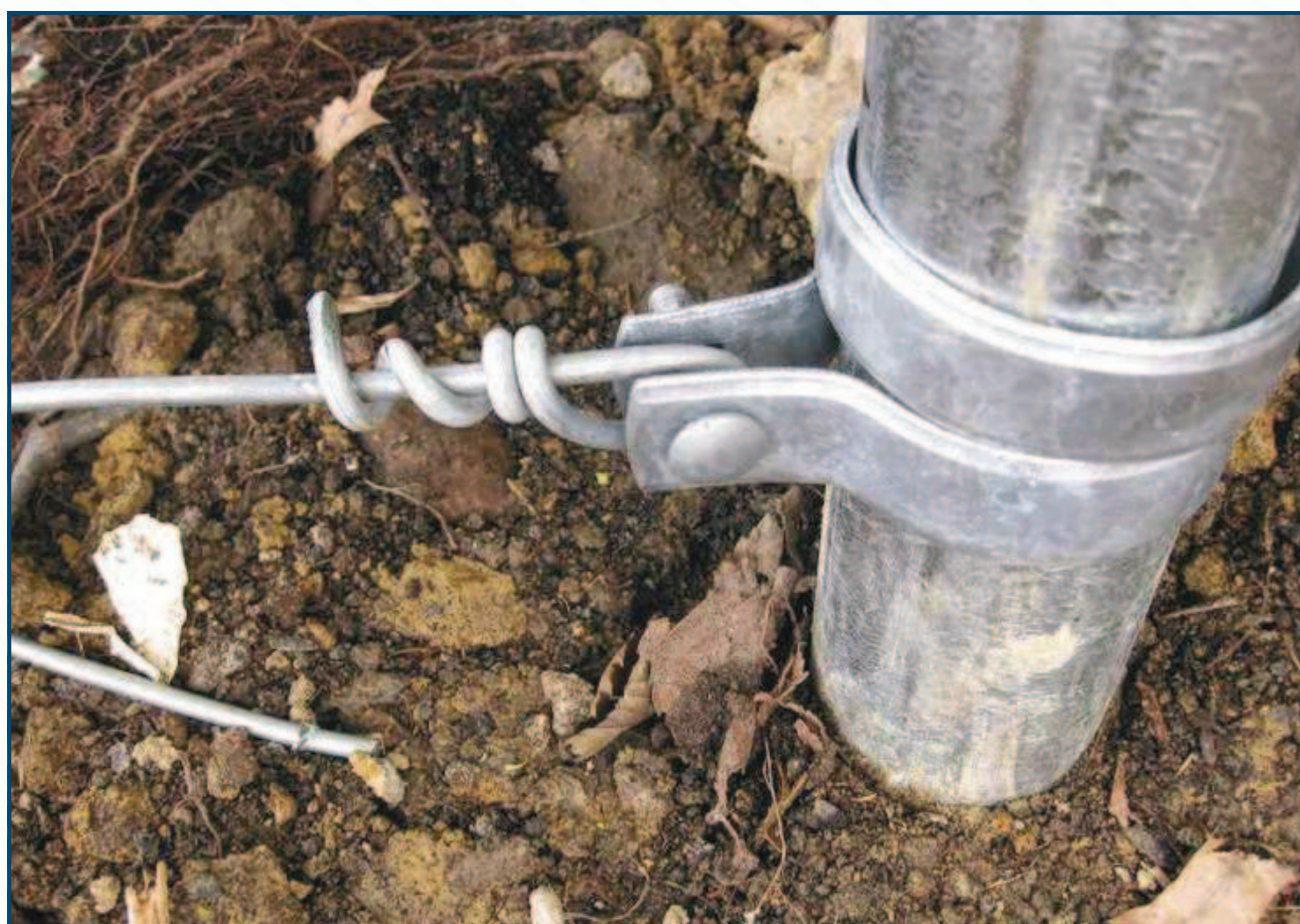
Tension band reinforces chain link fence
